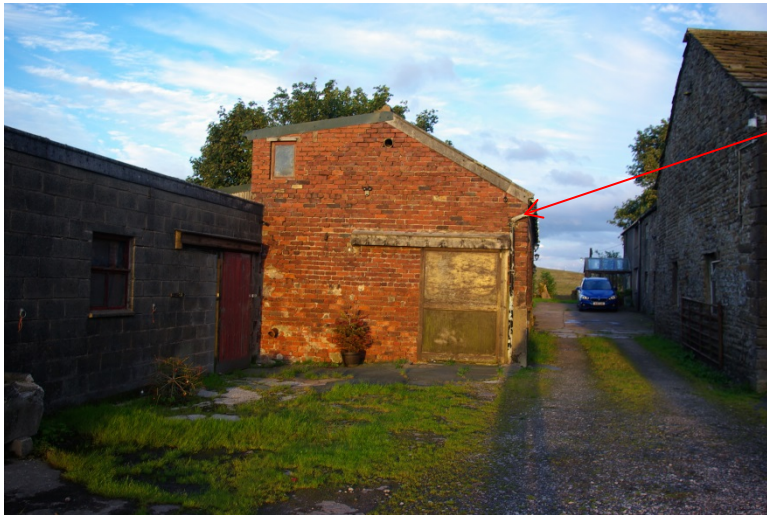
Building 5 - West Gaps behind verge caps
